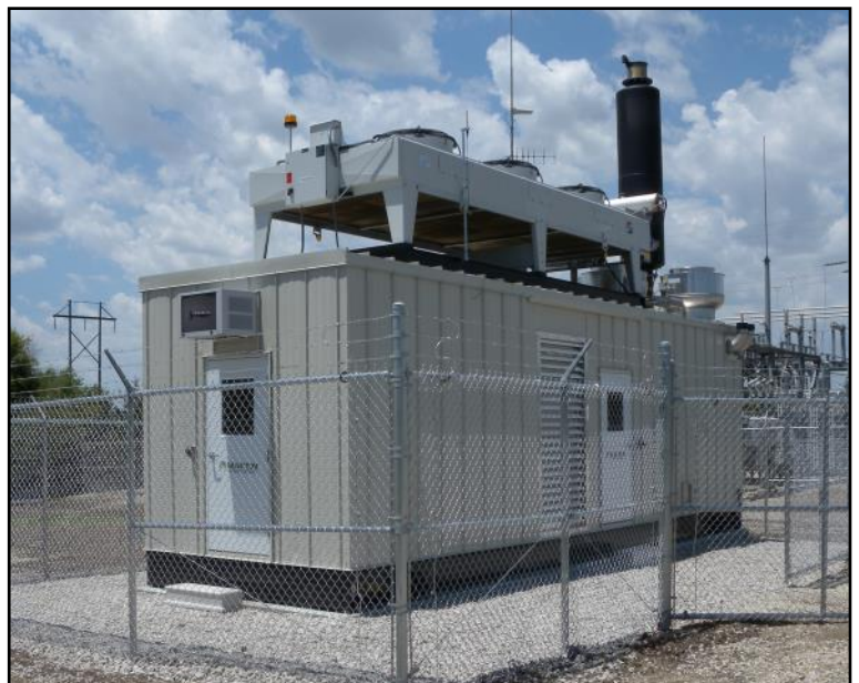
Butler Rural Electric Cooperative demand response generator
