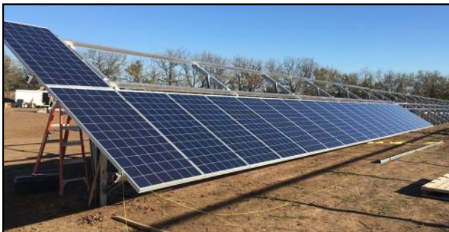
Installed solar panels
