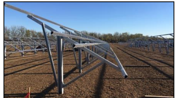
Solar panel racking system
